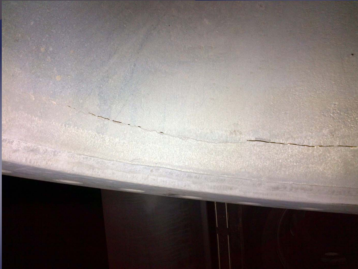
POE Monotube Cracks
