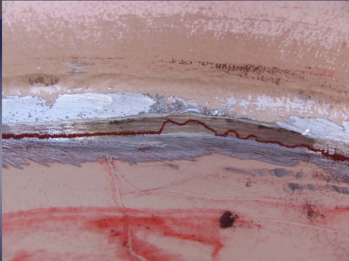
Western Monotube Crack
