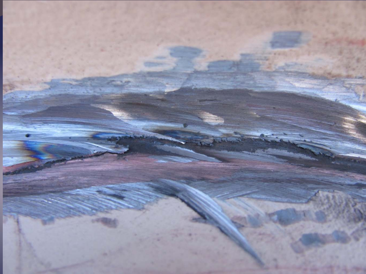
Western Monotube Crack
