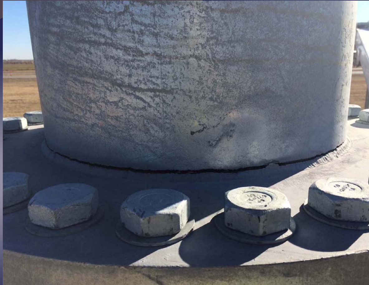
POE Monotube Cracks
